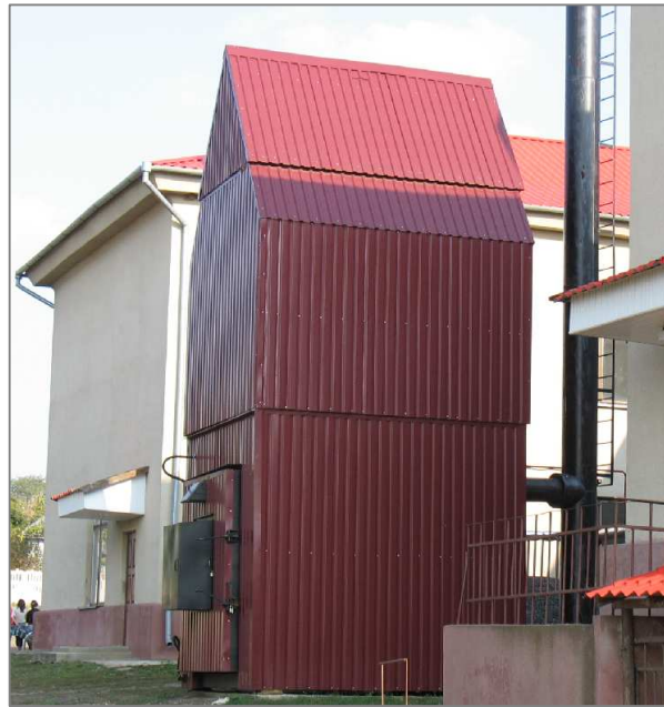
Biomass heating system (straw bale boilers) installed at a school in Taraclia village, Causeni raion.
