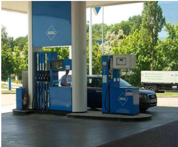
Dispensers integrated with the other fuels Jameln with Compressor Building in the back
