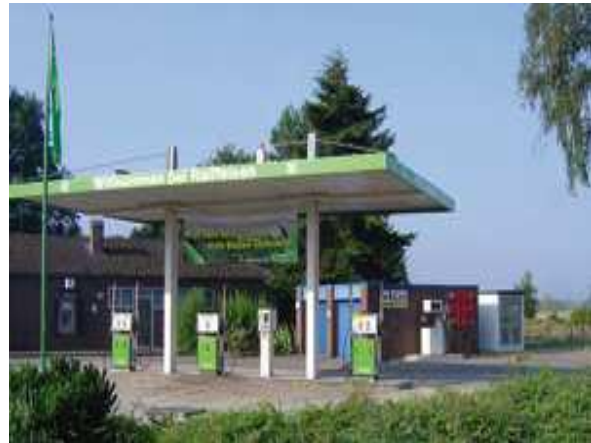
NGV/CNG Fuelling Station with Concrete Compressor Building on a conventional Fuelling Station with external Dispensers
