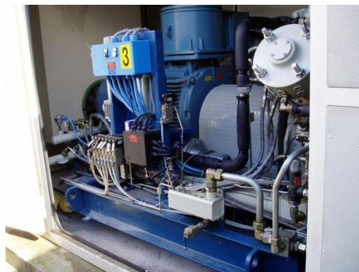
SAFE compressor of the Lille Bus depot
