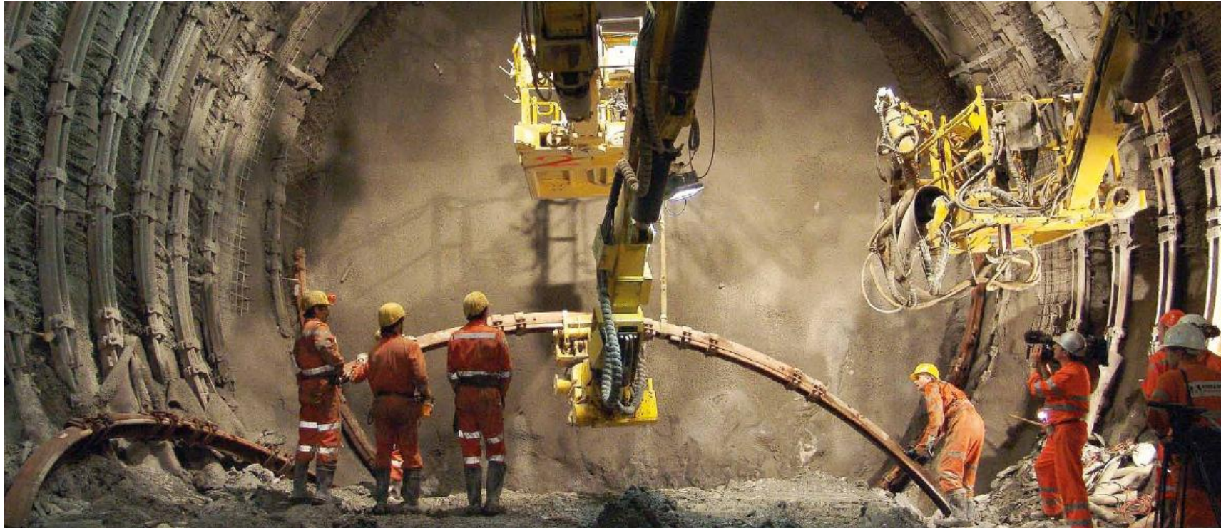
Tunnel workers at the Gotthard construction site of the new transalpine rail link.
