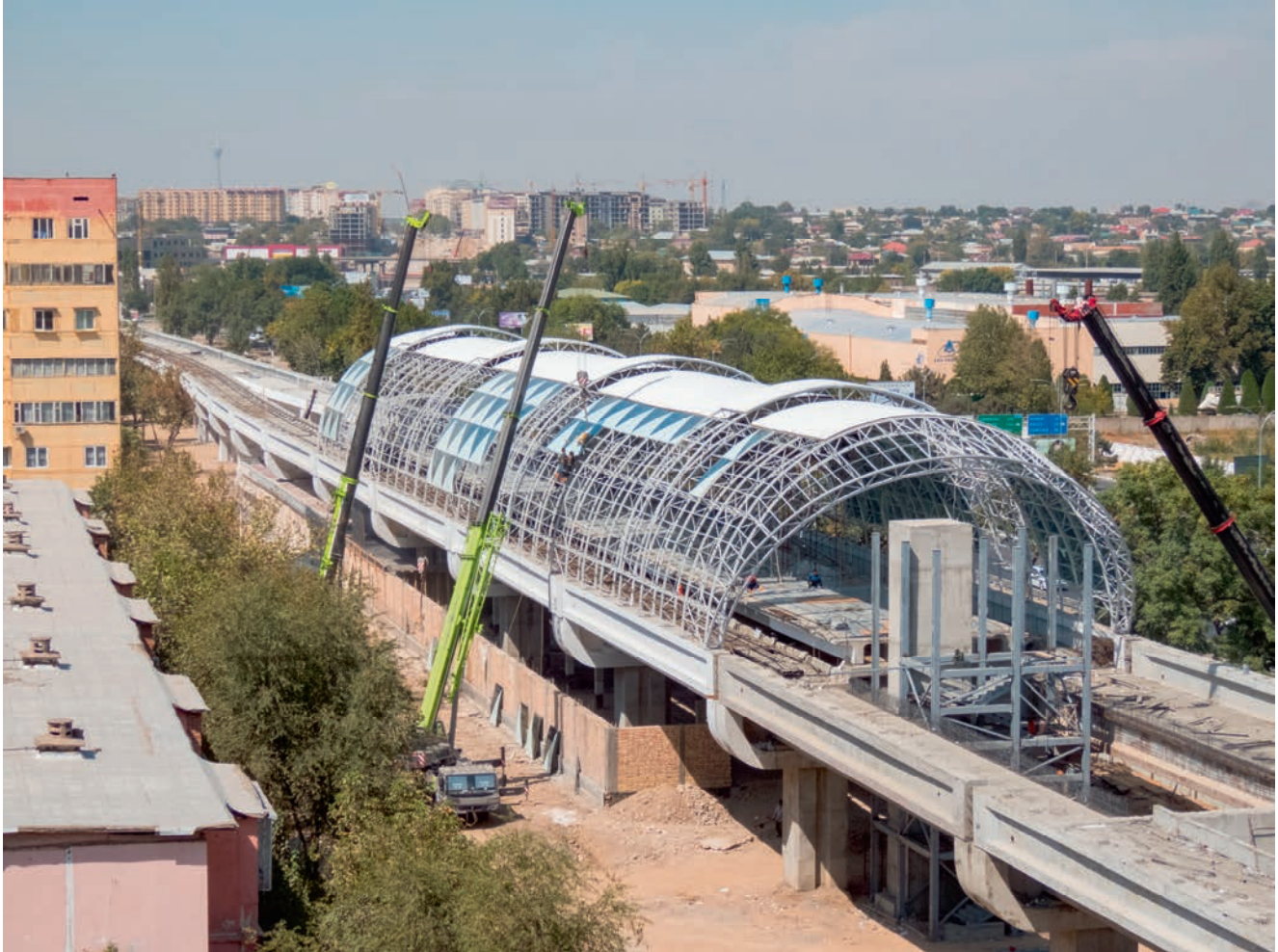
Photo 14.4: Construction of a new station for a surface line of Tashkent Metro along Akhangaran Road
