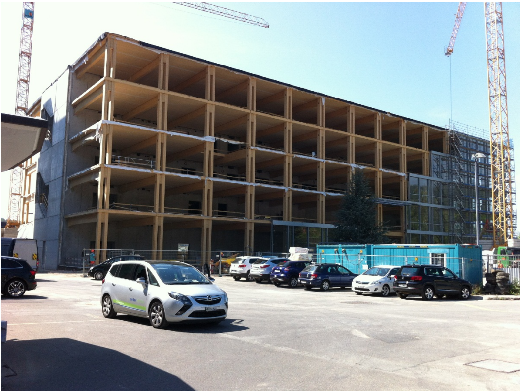
Fig. 8 – The shell of the Omega manufacturing building with partly cladded façade. (Image source: Eduard J. Belser, Egerkingen)
