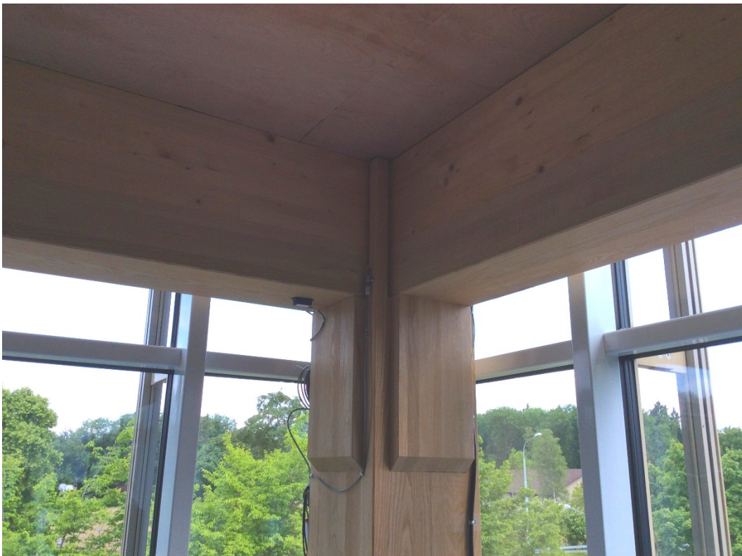
Fig. 3 Using a variety of sensors, the monitoring system, which is installed on the columns and beams, monitors and records the behaviour of the wood components of the post-tensioned glued-laminated hardwood timber frame. (Image source: Eduard J. Belser )
