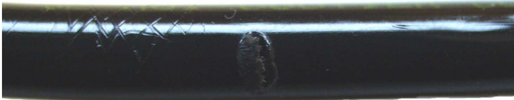
Fig.5: Electrical breakthrough of a plastic fuel line to a metal clamp at 3 kV
