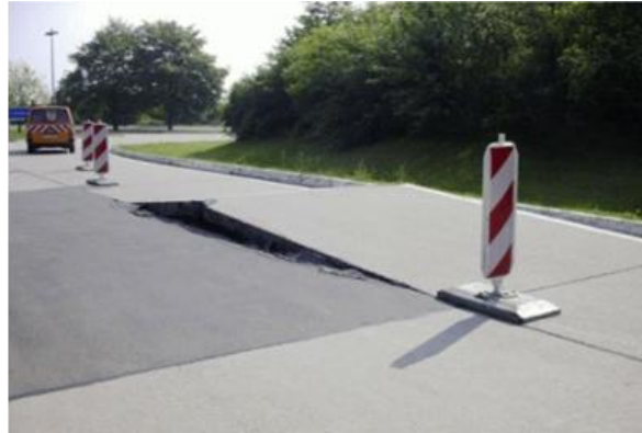
More "Blow ups" in concrete surfaces
