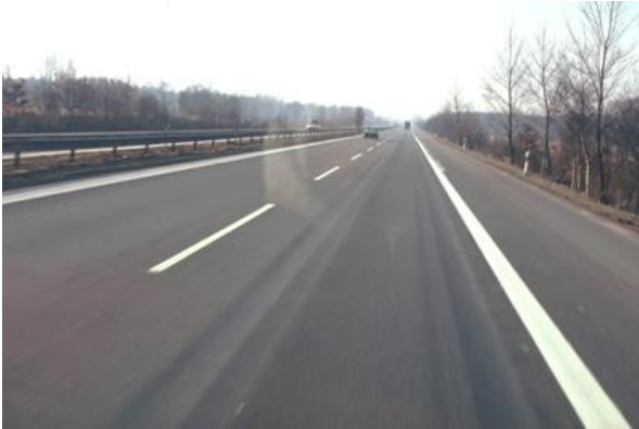
Increase in rutting
