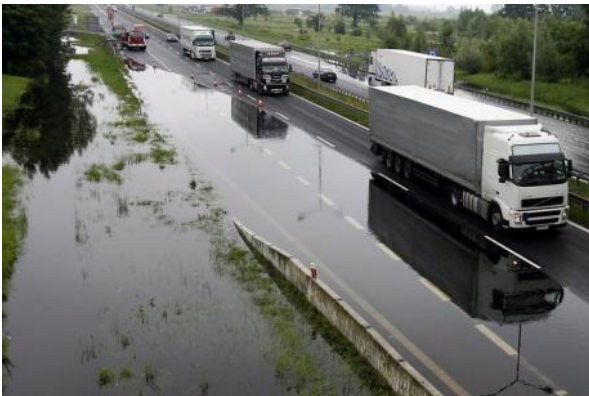
Inundation due to ill-dimensioned drainage systems
