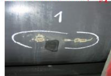
Corrosion initiation ( Type 1)
