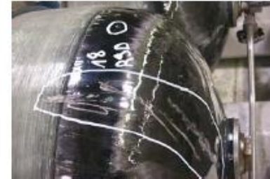
Deep scratches damages
