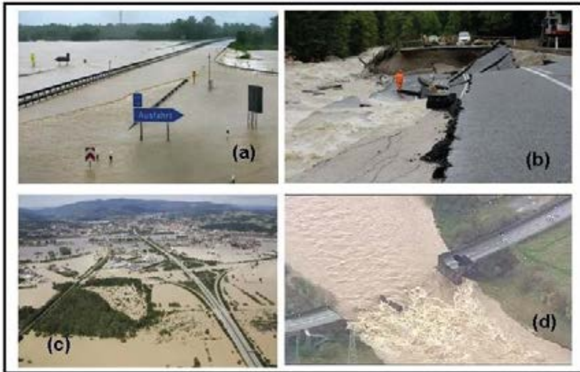
Figure 26 Flood damages on roads (a) Highway 8 (Munich to Salzburg) in Grabenstaett near Traunstein, S. Germany (early June 2013, Matthias Schrader, AP); (b) heavily damaged road between Lofer and Waidring in Tyrol (Austria) (3rd June, 2013, Kerstin Joensson, AP); (c) flooded highways in Deggenfendorf; and (d) collapsed bridge in Cumbria ( United Kingdom of Great Britain and Northern Ireland) in November 2009, ( http://news.bbc.co.uk/2/hi/uk_news/8369934.stm ).
