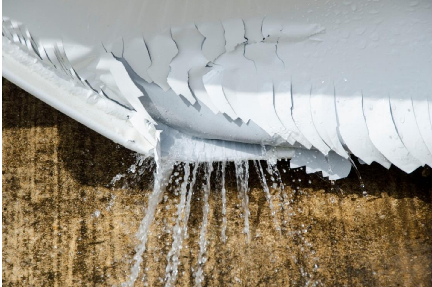
2011 - leak at the top of the impact area – front end dish
