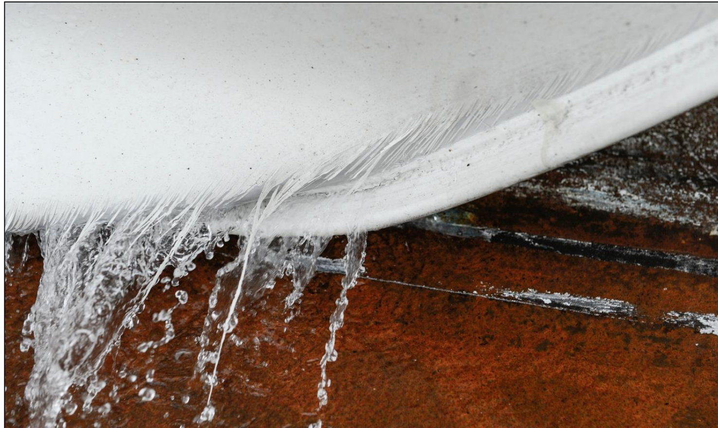
2008 - leak at the top of the impact area – rear end dish
