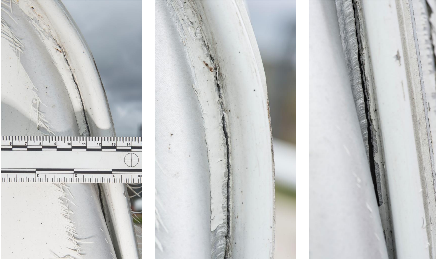
2008 - rupture within the fillet weld between the rear end dish and extrusion band at the top of the impact area
