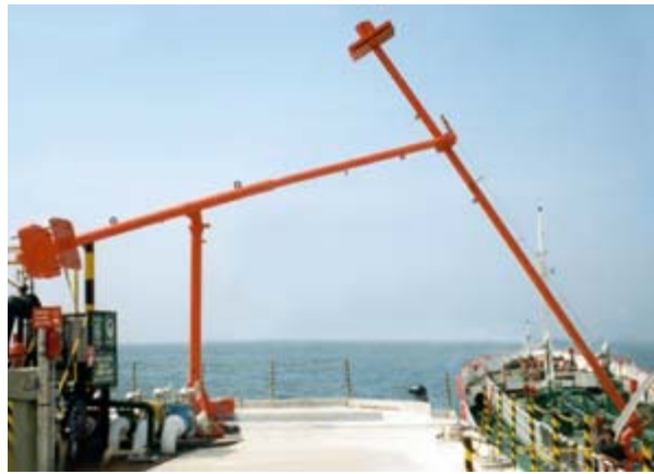
Figure 3 Loading arm being used to transfer fuel to a waiting barge.
