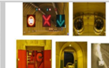
TUNNEL CONTROL SYSTEMS
