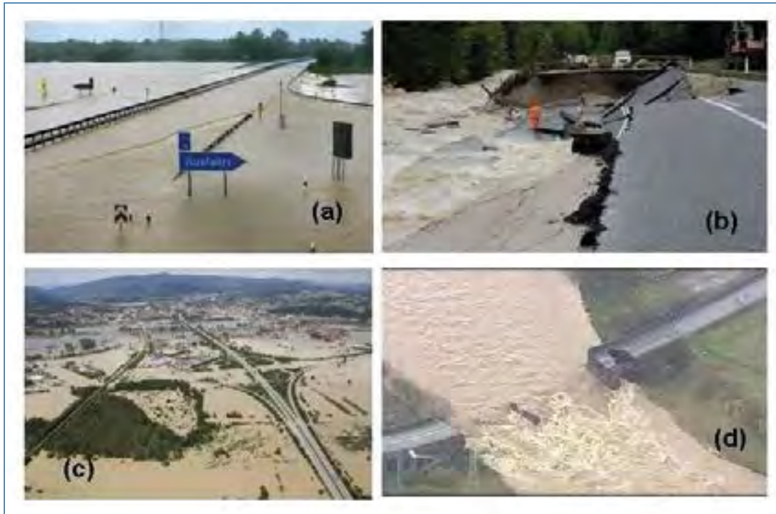
Figure 26 Flood damages on roads (a) Highway 8 (Munich to Salzburg) in Grabenstaett near Traunstein, S. Germany (early June 2013, Matthias Schrader, AP); (b) heavily damaged road between Lofer and Waidring in Tyrol (Austria) (3rd June, 2013, Kerstin Joensson, AP); (c) flooded highways in Deggenfendorf; and (d) collapsed bridge in Cumbria ( United Kingdom of Great Britain and Northern Ireland) in November 2009, ( http://news.bbc.co.uk/2/hi/uk_news/8369934.stm ).
