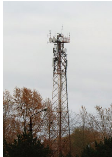
Telecommunications, RIS and VTS tower on the river Sheksna (the Russian Federation).
