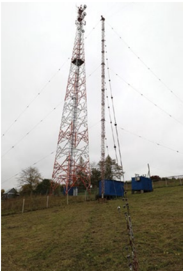
Telecommunications tower and the GNSS reference station near the village of Ivanov Bor on the river Sheksna (Russian Federation).
