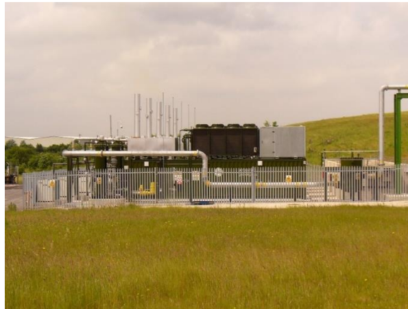
Figure 9.6 Harworth Colliery gas engines
