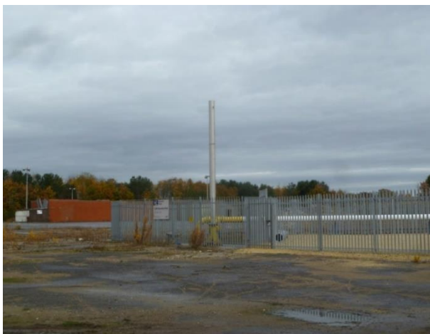
Venting arrangement at the Stillingfleet Mine
