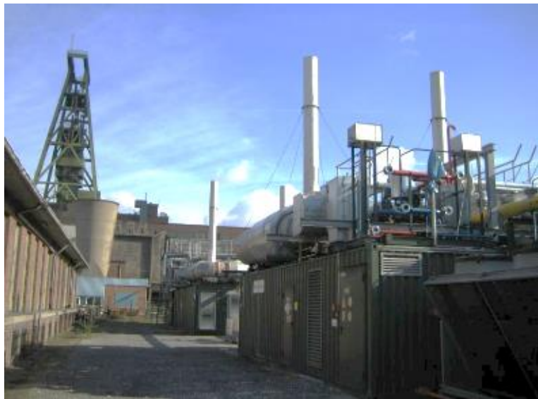
Figure 9.2 Lohberg Power Generation Station
