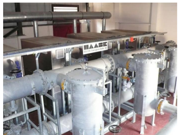
Stillingfleet Mine gas extraction plant
