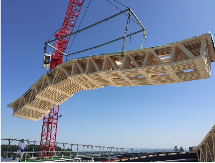
Fig. 10 Mounting of the roof of the Arch-Tec-Lab at the Institute of Technology in Architecture (ITA) (Image source:ETH/ITA Zurich)
